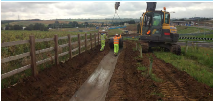
Lining the bottom of the transverse with the first longitudinal layer of CC
