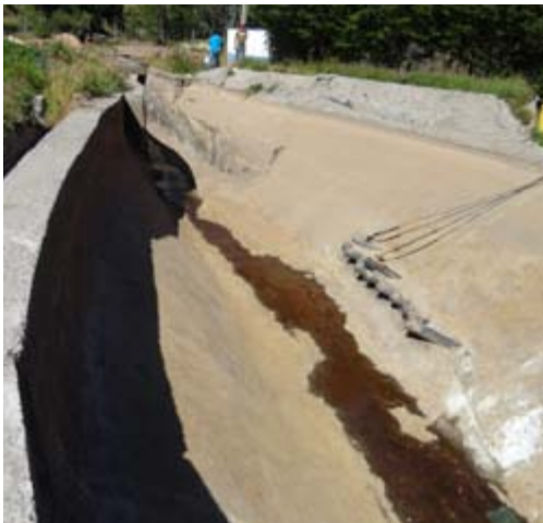
Dilapidated concrete reservoir
