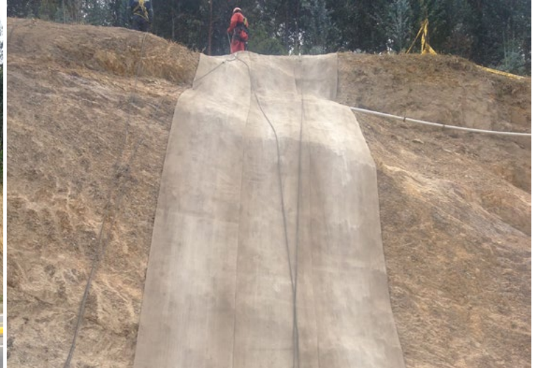
A spreader beam and climbing equipment was used to lay lengths of CC5
