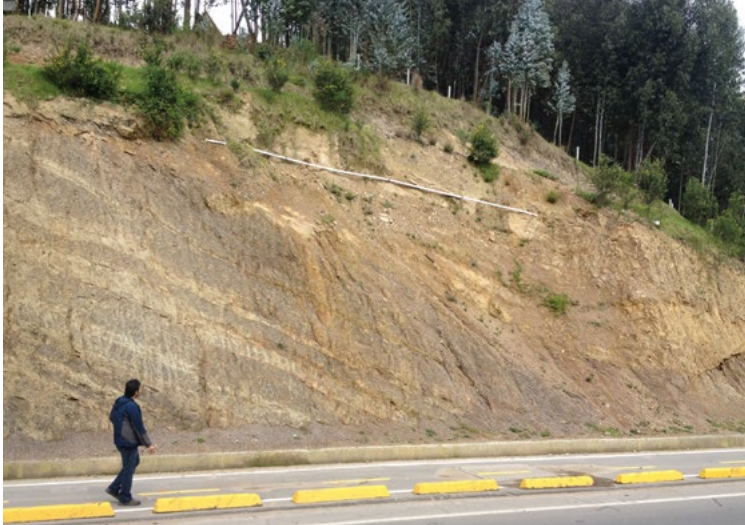
The slope prior to installation of CC, displaying signs of slip and erosion
