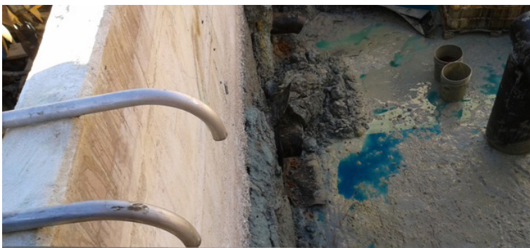
Dilapidated concrete acid tank (in disrepair due to many years of exposure)
