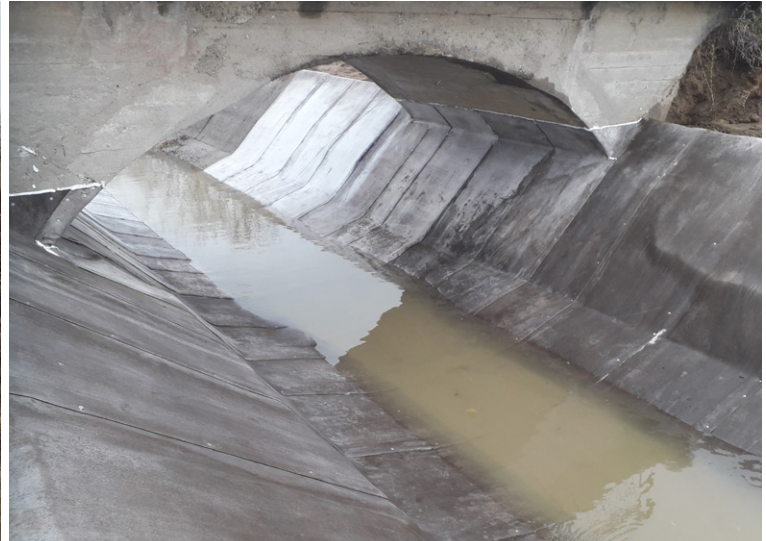
CC termination around bridge
