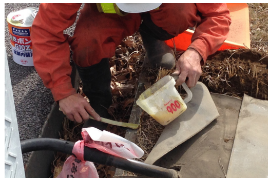
CC was cut to fit around the pipes and glued in place
